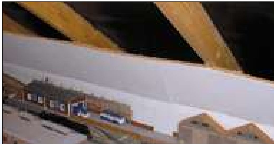
Picture 2 Mould on rafters evident due to misuse of roofspace by tenant blocking ventilation
