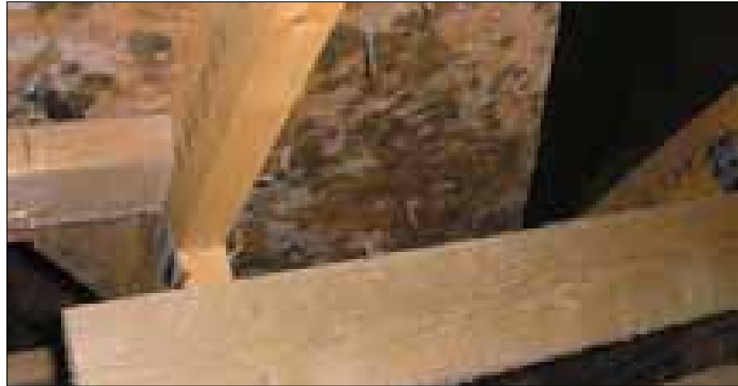
Picture 1 Mould is evident on Timber Boarding due to vapour unable to escape in dormer detail
